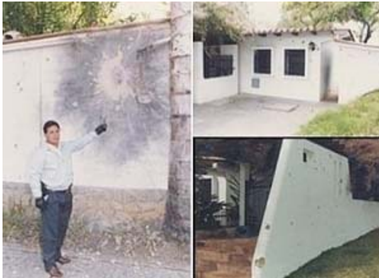
Damaged caused by the attacks against the Venezuelan White House during the failed coup d'état directed by Chavez en 1992
